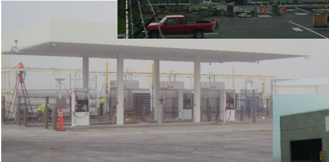
CNG Fueling Facility
